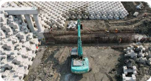
● Concrete Block Groundsill Cipamingkis River
